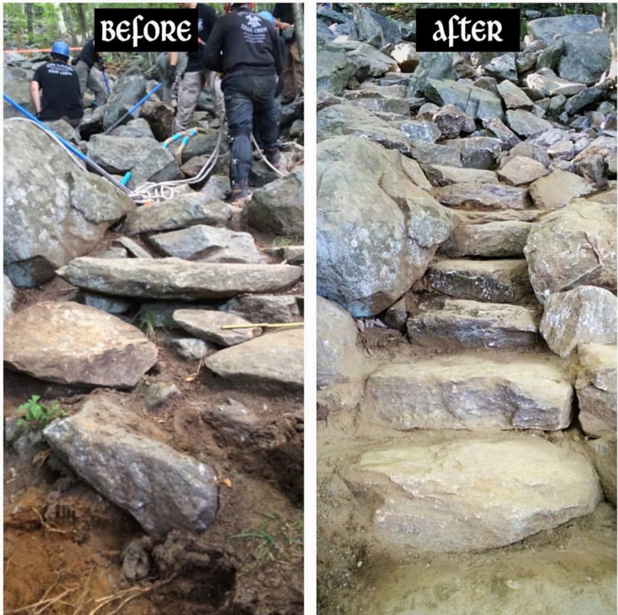
Before and after shots of a previously unsafe trail stretch converted to steps.
